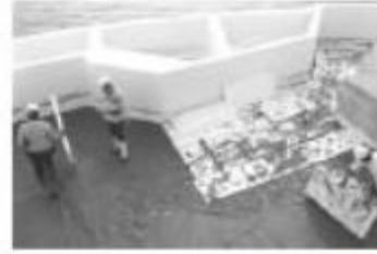
Fig. 6.2—EPS insulation board placed in cellular concrete slurry over structural concrete deck.
