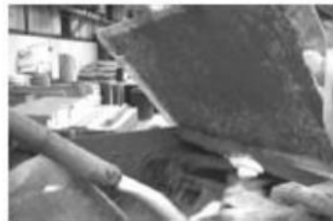
Fig. 2.2—Metering preformed foam into cement-water slurry (click on picture to view video).
