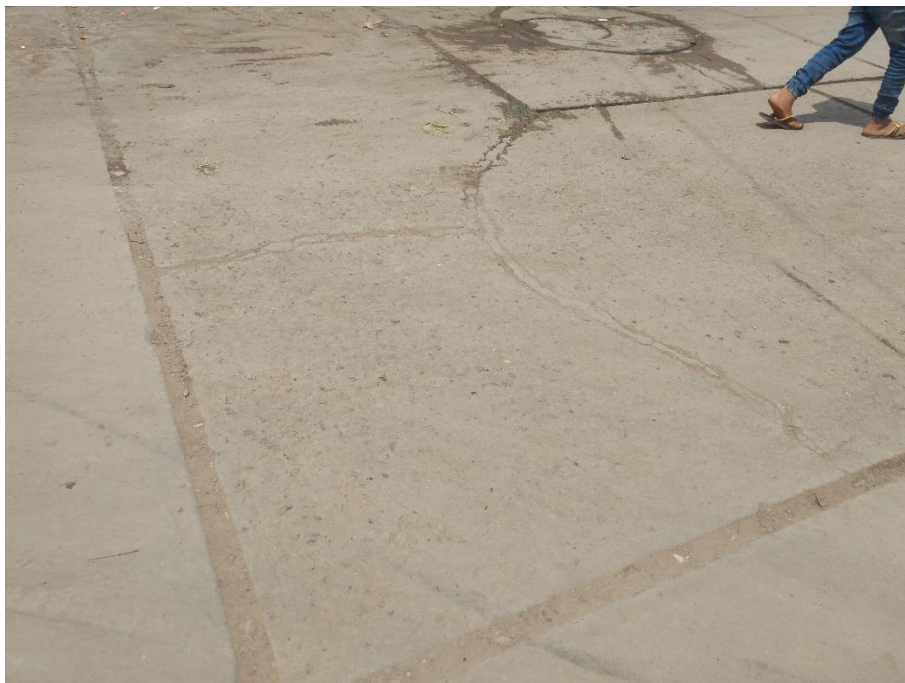
Figura 28: fisura transversal o diagonal
