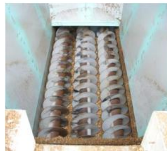
Mounting in discharge screw (wood-fired power plant)
