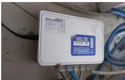
Figura 8: switch no administrables
