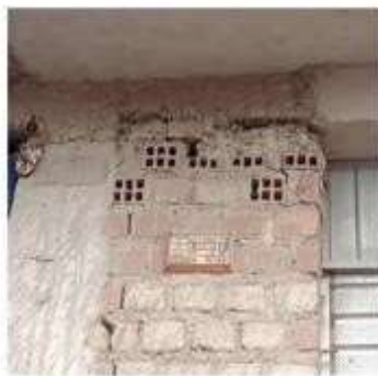
Mala union muro - techo
