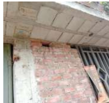
Mala union muro-techo
