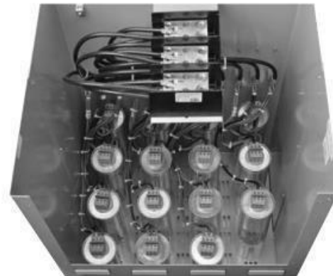
Unipak interior—E1 enclosure
