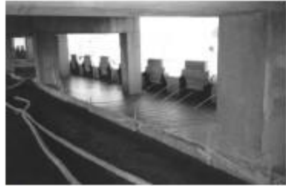
Fig. 7.1—Geotechnical application under a bridge structure with mechanically stabilized earth (MSE) containment walls.
