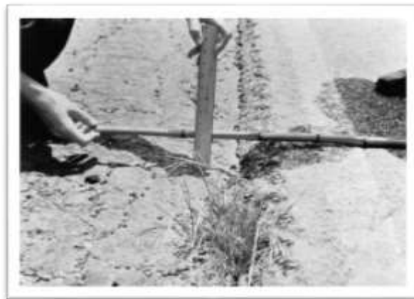
Figura 28: Desnivel carril/berma, severidad media
