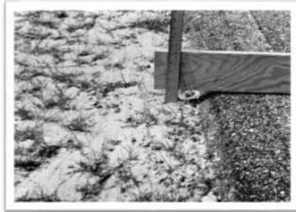
Figura 27: desnivel carril/berma, severidad baja
