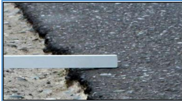
Figura 23: Desnivel Carril Berma
