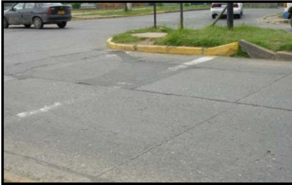
FIGURA 8 Falla de blowup – buckling
